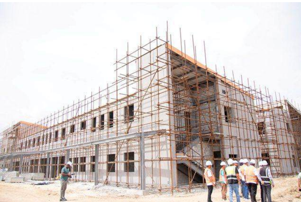
Construction of the new Lima Hospital, Essequibo Coast in Region Two (Pomeroon-Supenaam).
